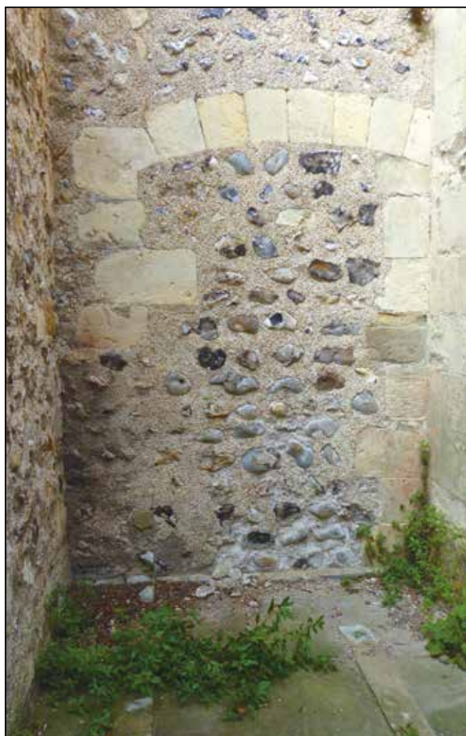
Possible Saxon doorway discovered in the 1936 restoration (see page 114), seen on the South side of the chancel, between a buttress and the boiler room
