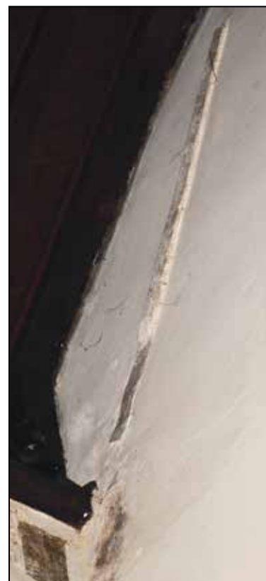
The old steeper roofline can be seen above, on the tower wall facing west
