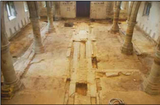
A view possibly not seen since the 1500s before the first box pews began to be installed. This is how the nave looked after the pews had been removed.
