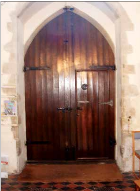
The inner west doors which probably dated from the 1862 restoration and were removed in 2009
