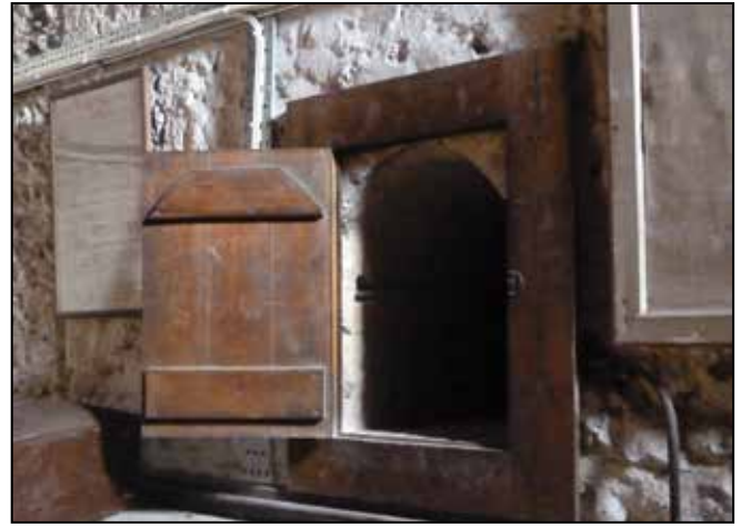
Door in the east wall of the ringing loft giving access to the space above the ceiling of the chancel
