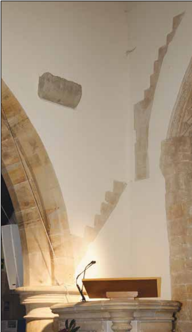
The stone buttresses above the pulpit for supporting the rood. The outline of the steps can also be seen.
